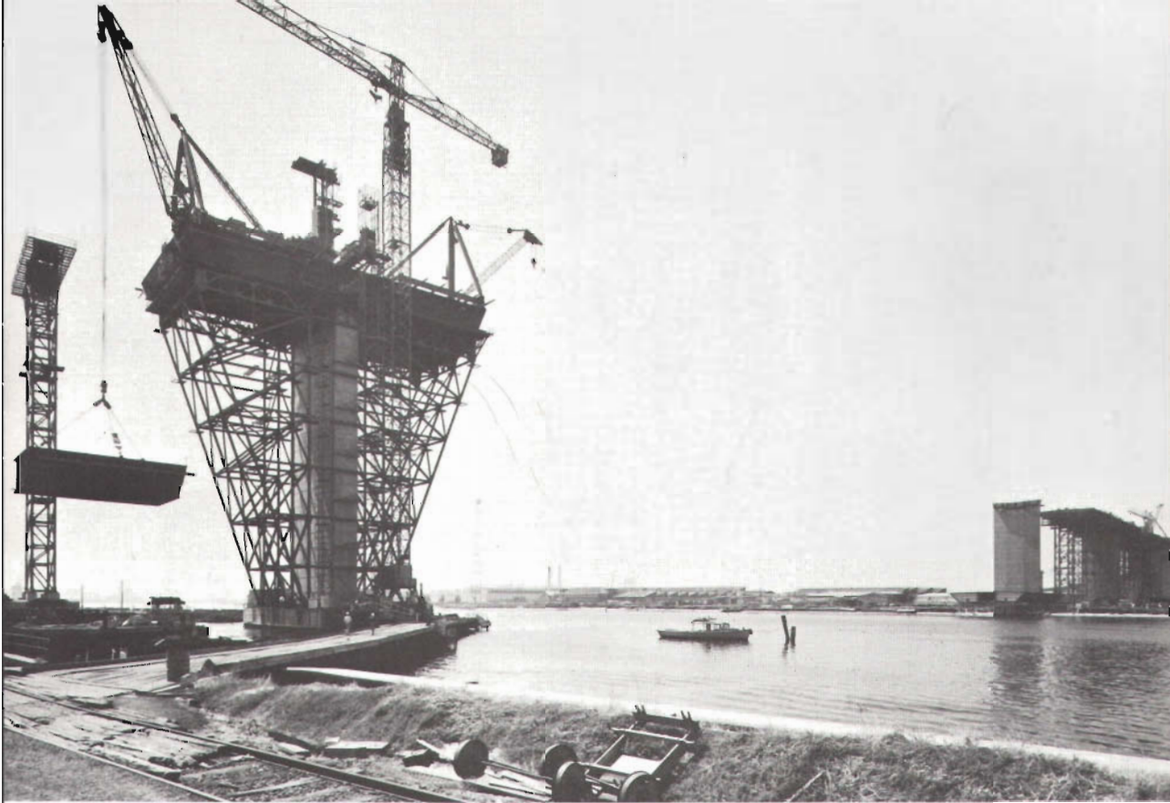
A general view of the crossing place showing, at left, the West Main Pier, and, at right, the steel spans on the east bank of the Yarra River.
