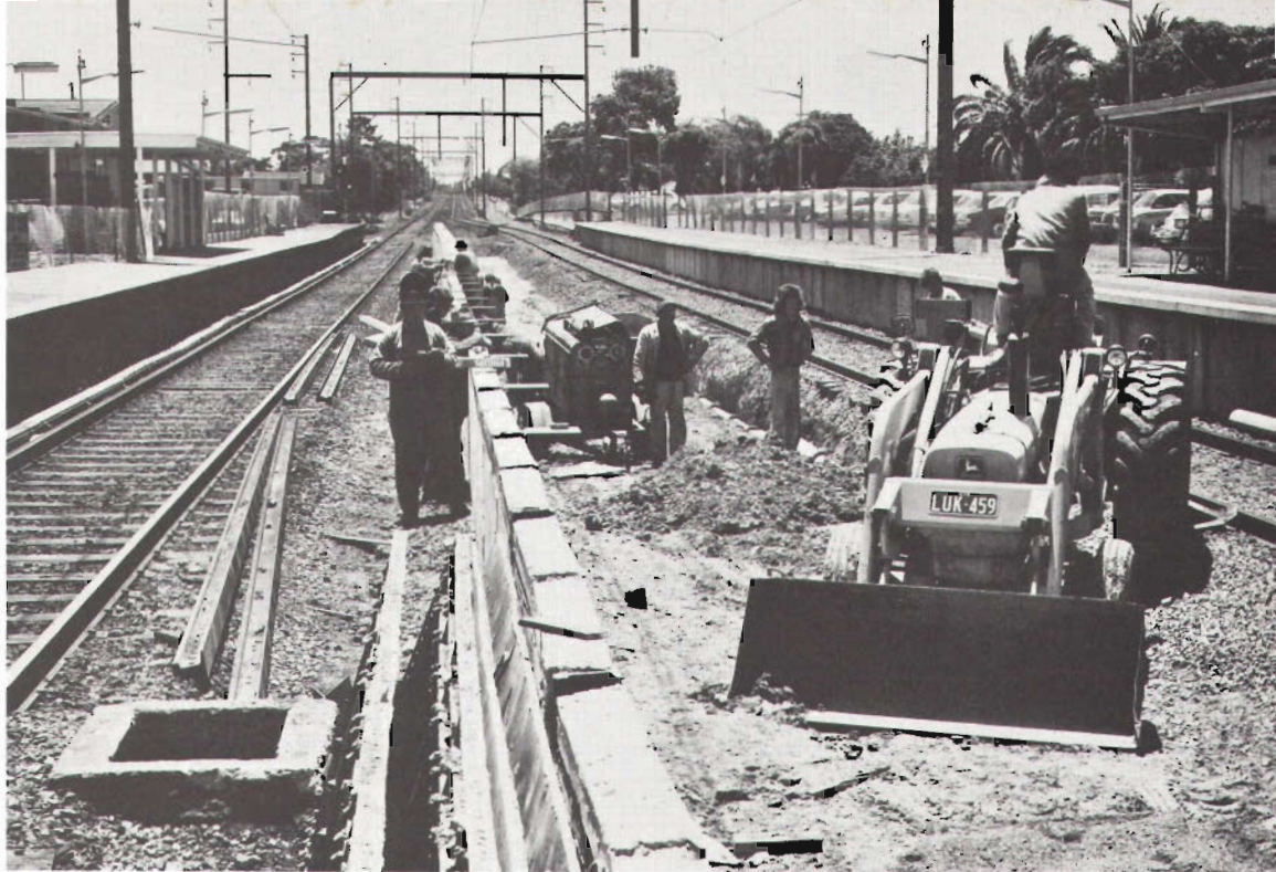
Track duplication work in progress near Ormond railway station—part of an extensive track upgrading programme with the Victorian Railways. Victorian Railways Board
